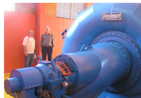
Elemar Battisti with Francis turbines Usina Granja Velha.
