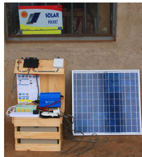
Solar 'power station' at a retailers in Tororo.
